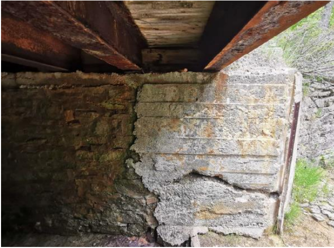
Fair Condition Abutment Wall Extension
