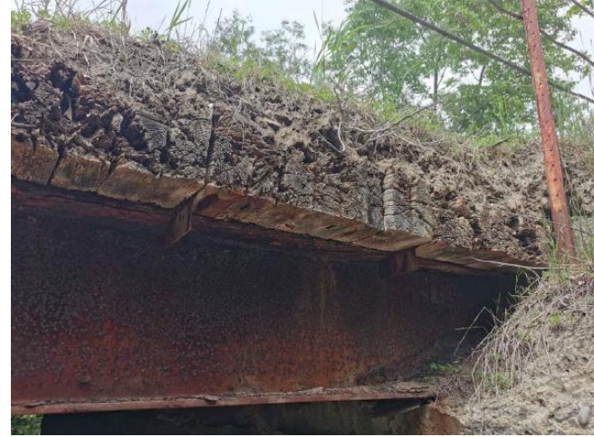
Poor Condition Deck
