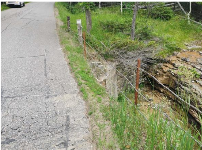
Poor Condition Guiderail
