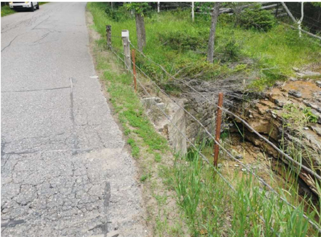
Poor Condition Guiderail
