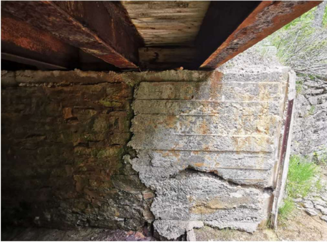
Fair Condition Abutment Wall Extension
