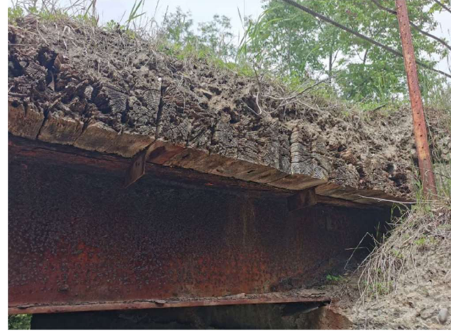
Poor Condition Deck
